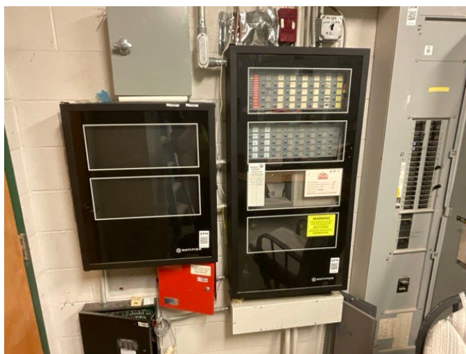
21 - FIRE ALARM PANEL
