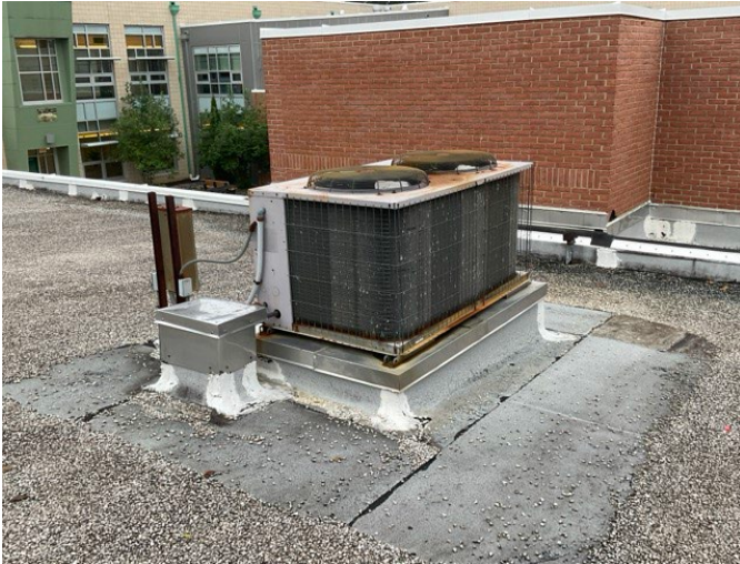
13 - SPLIT SYSTEM CONDENSER
